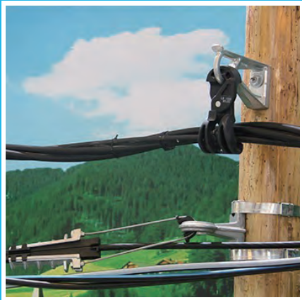
LV-ABC lines with insulated neutral messenger
