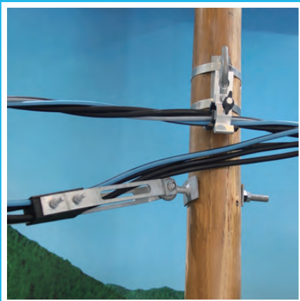
Self-supporting LV-ABC lines
